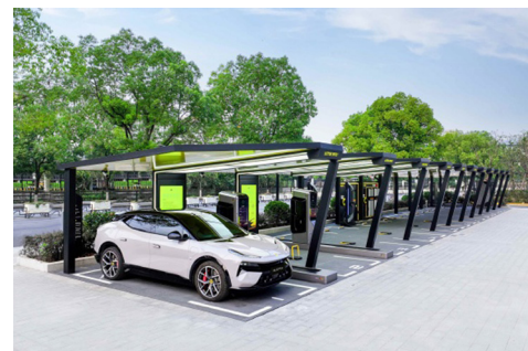
A Lotus charging station in China
