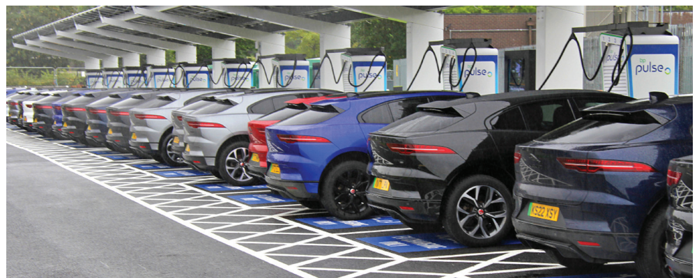
A fleet of 32 Jaguar I-PACEs were simultaneously used at the NEC facility to test the infrastructure in terms of power distribution, rapid charging and vehicle connection.
