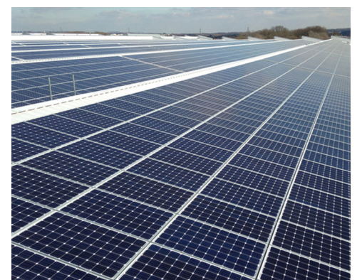
Existing Jaguar Land Rover solar rooftops will be expanded at all UK sites.
